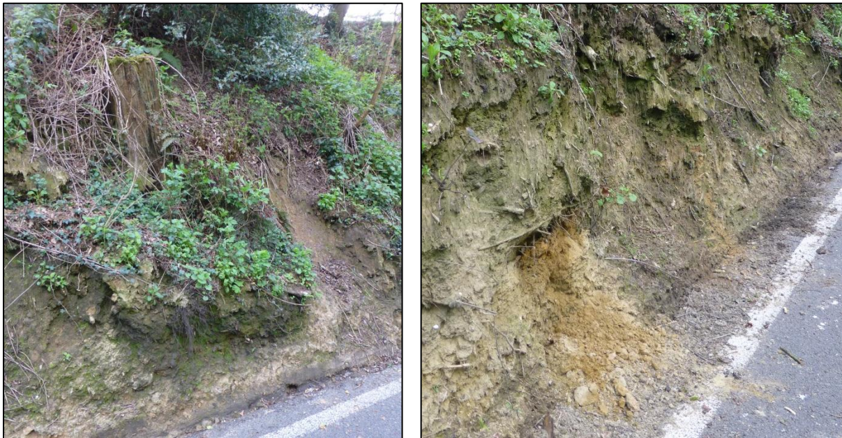
Figure 6: Shallow, Local Instabilities on Eastern Slope
