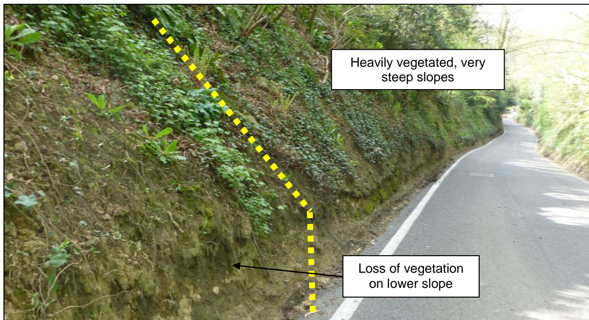
Figure 5: Eastern Slopes showing Signs of Undermining
