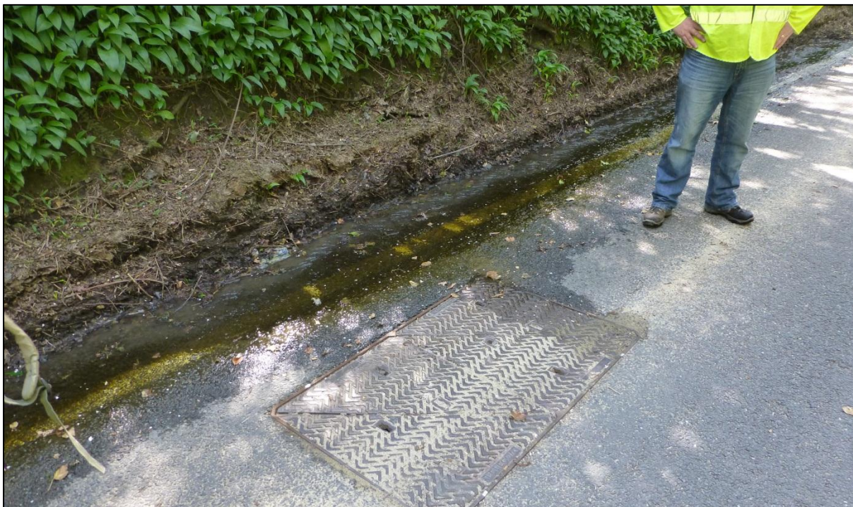
Figure 13: Seepage Running along Eastern side of Carriageway
