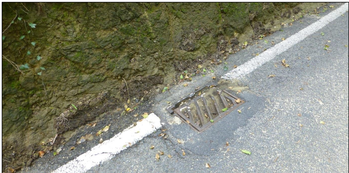
Figure 9: Blocked drain within Carriageway
